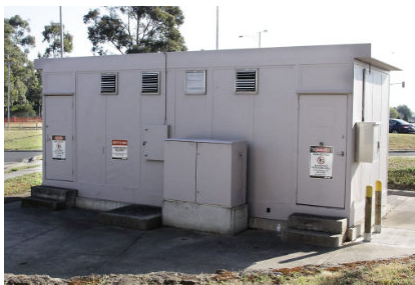
Tramway substation at the intersection of Kingsbury Drive and Plenty Road, 2012. Its compact size contrasts with the larger substation buildings on older parts of the network. Photograph by Marcus Wong.
